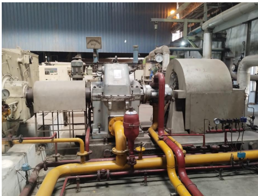
Figure 4: An image of a turbo-generator within the plant
